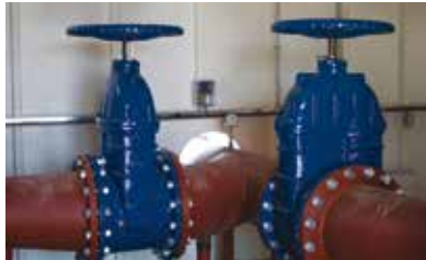
Pumps and Valves
